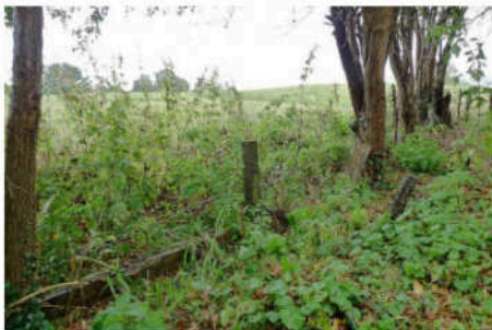
Repairing the perimeter fence to keep cattle out of the mill grounds
